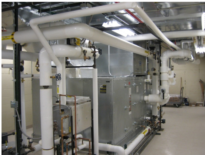
Figure 1.2 – Air Handler Unit
